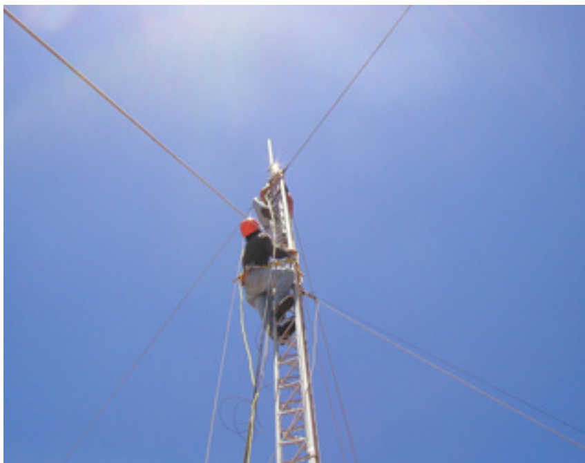
Figure 8.2: A climbable guyed tower.
